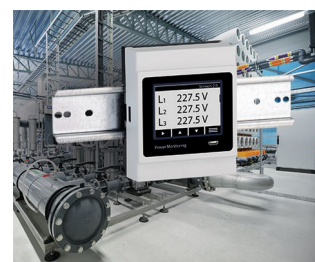
Monitoring of electrical variables
