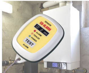
CO Gas Alarm
